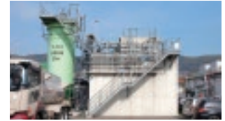
Water treatment equipment
