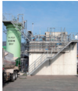
Water treatment equipment
